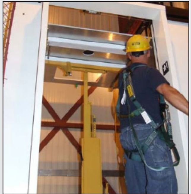
Long cord on the remote pendant station allows the installer to stand outside the hoistway as the canopy is being lifted into position.
