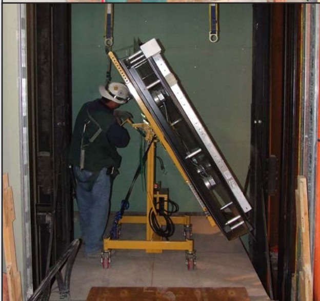
One worker can maneuver loaded lift to safely and rapidly raise the canopy assembly into place.
